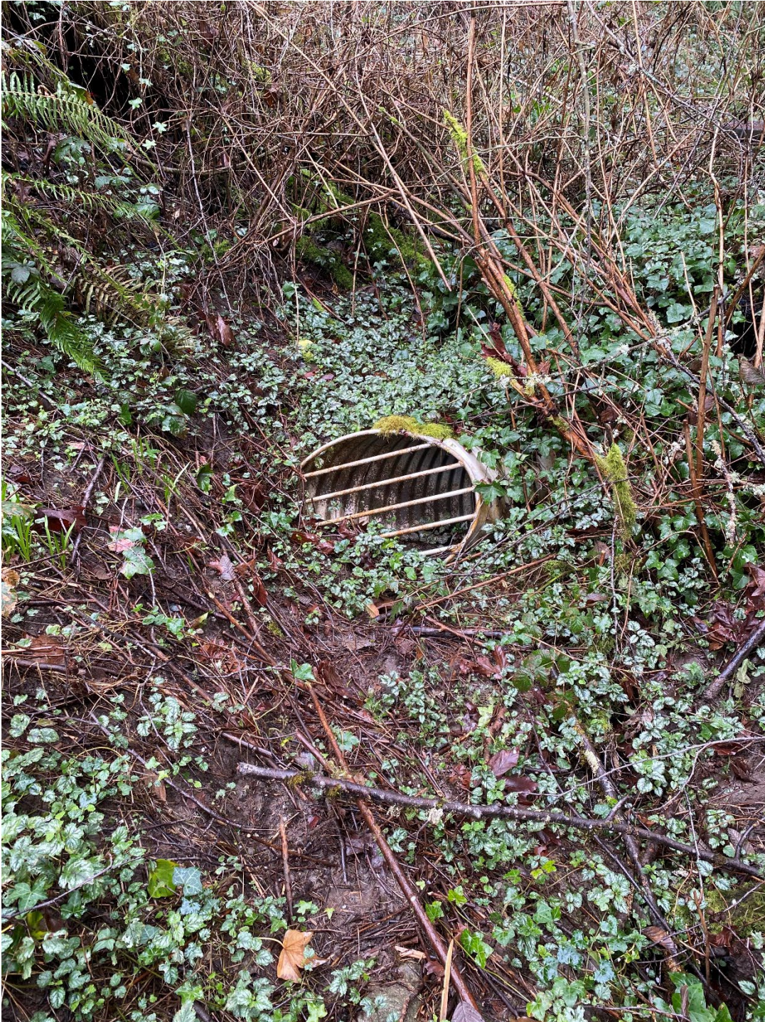
View of culvert at bottom of ravine. Note no surface channel or flow entering culvert. Running water could be clearly heard beneath the surface within likely piped watercourse.
